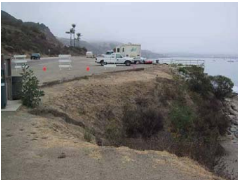
Evidence of bluff erosion adjacent to Avila Beach Drive, across from Harbor Terrace.
